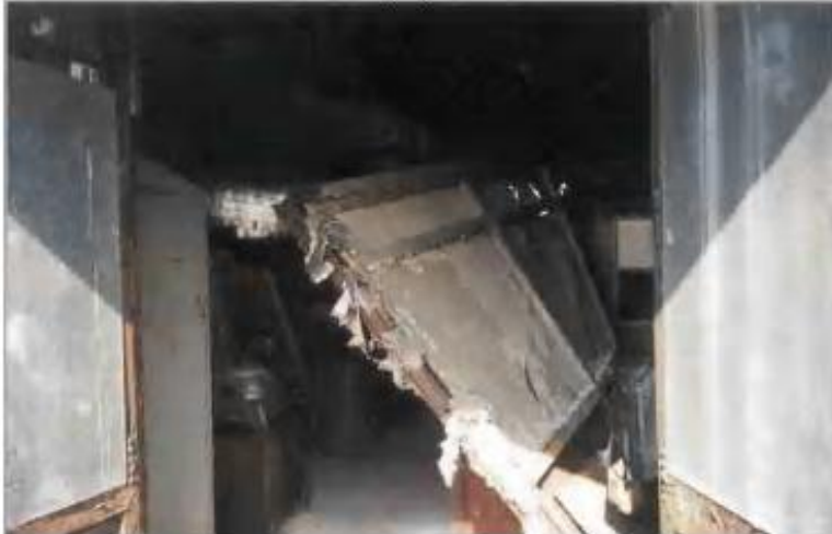
Cracked and torn partition in a condemned section of the Support Service Division storehouse.
